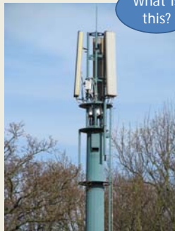
It is a mobile phone mast
